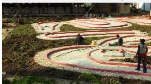
Msasani Sports Facility Mini Golf Construction underway. By Landscape Architect Carolyn Wanza of Ecoarch Solutions Ltd. (Nairobi)
